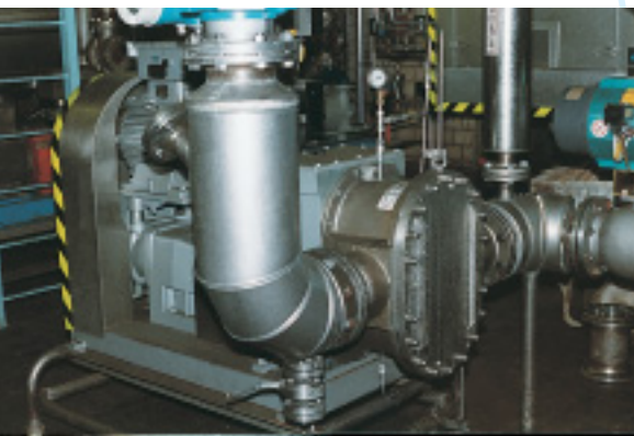
FKL for transfer of paint and glue dispersion at Hoechst, Frankfurt.
